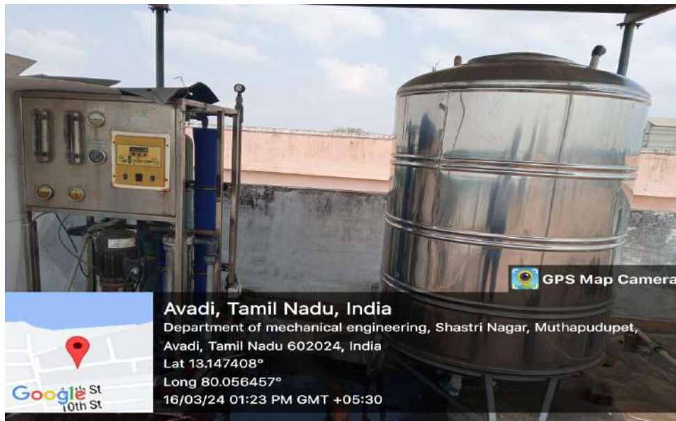
RO Plant Located in Mechanical Engineering Block
