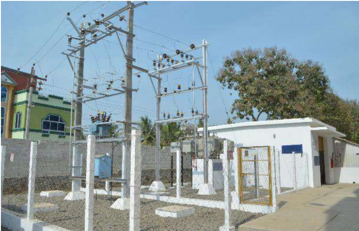
11 kV/415 V HT Substation
