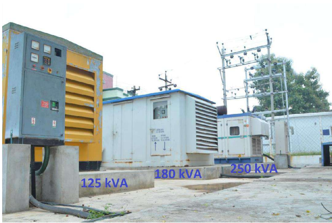
Kirloskar Diesel Generator (3Nos) installed in our College Campus for Backup Electric Supply
