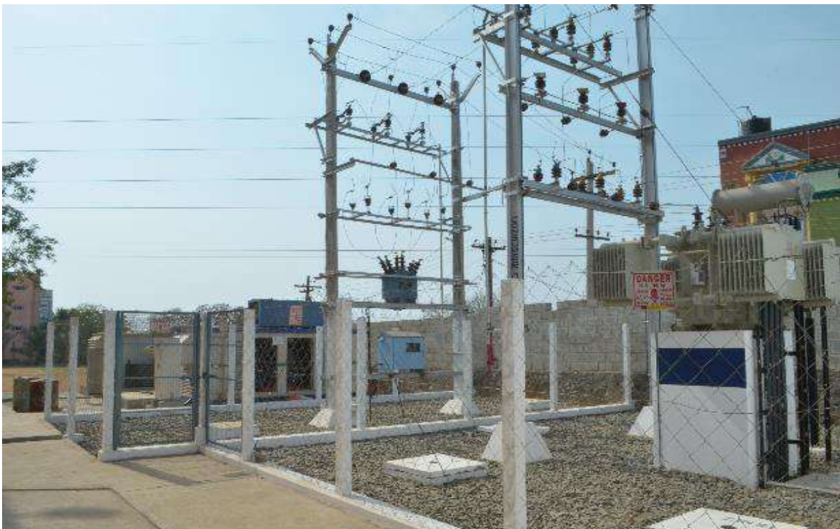
11 kV/415 V HT Substation
