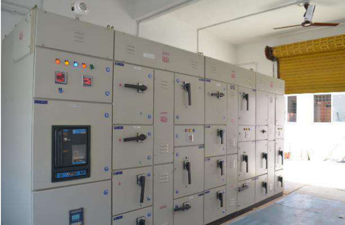
HT Substation Control Room
