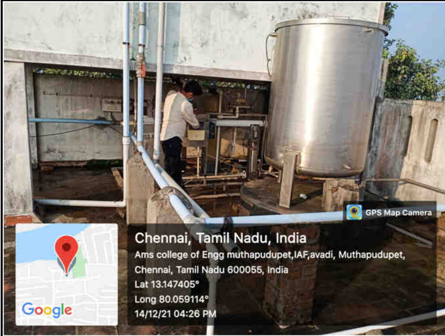
Figure 9.3.3 R-O WATER PLANT Facilities with a capacity of 500 l/hr.
