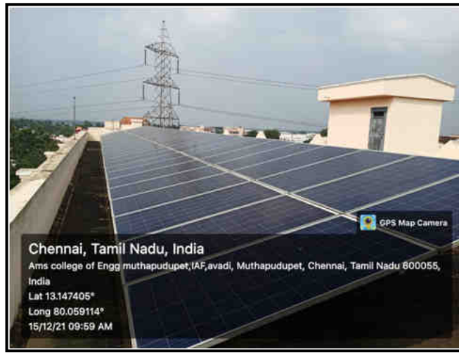
Figure 9.3.2 20 KW Rooftop Solar Panel
