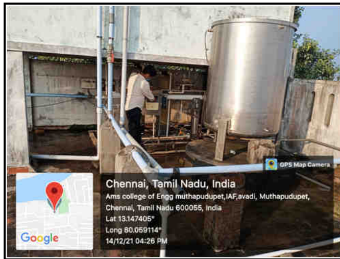
Figure 9.3.3 R-O WATER PLANT Facilities with a capacity of 500 l/hr.
