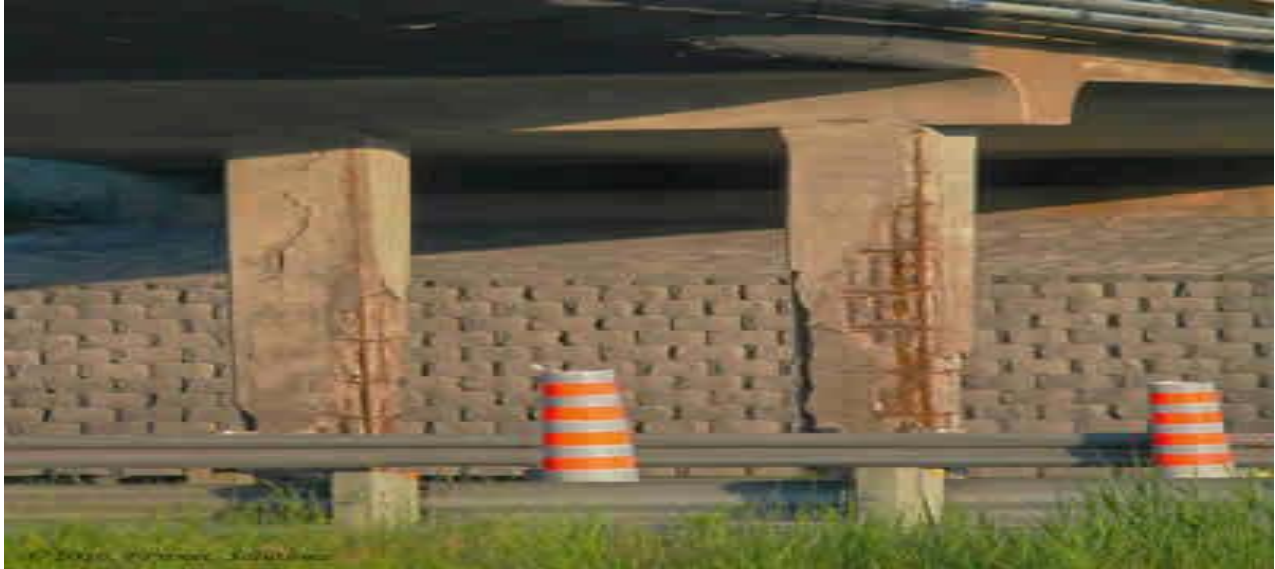
Structural Effects of Corrosion
