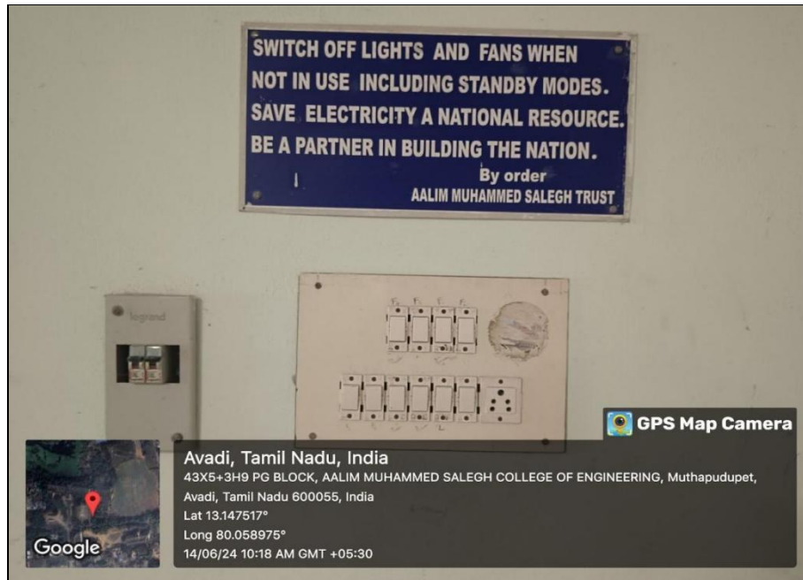
Figure: Save Electrical Energy Sign boards in appropriate places
