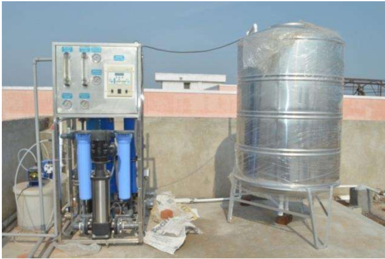
RO Plant Installed in the campus
