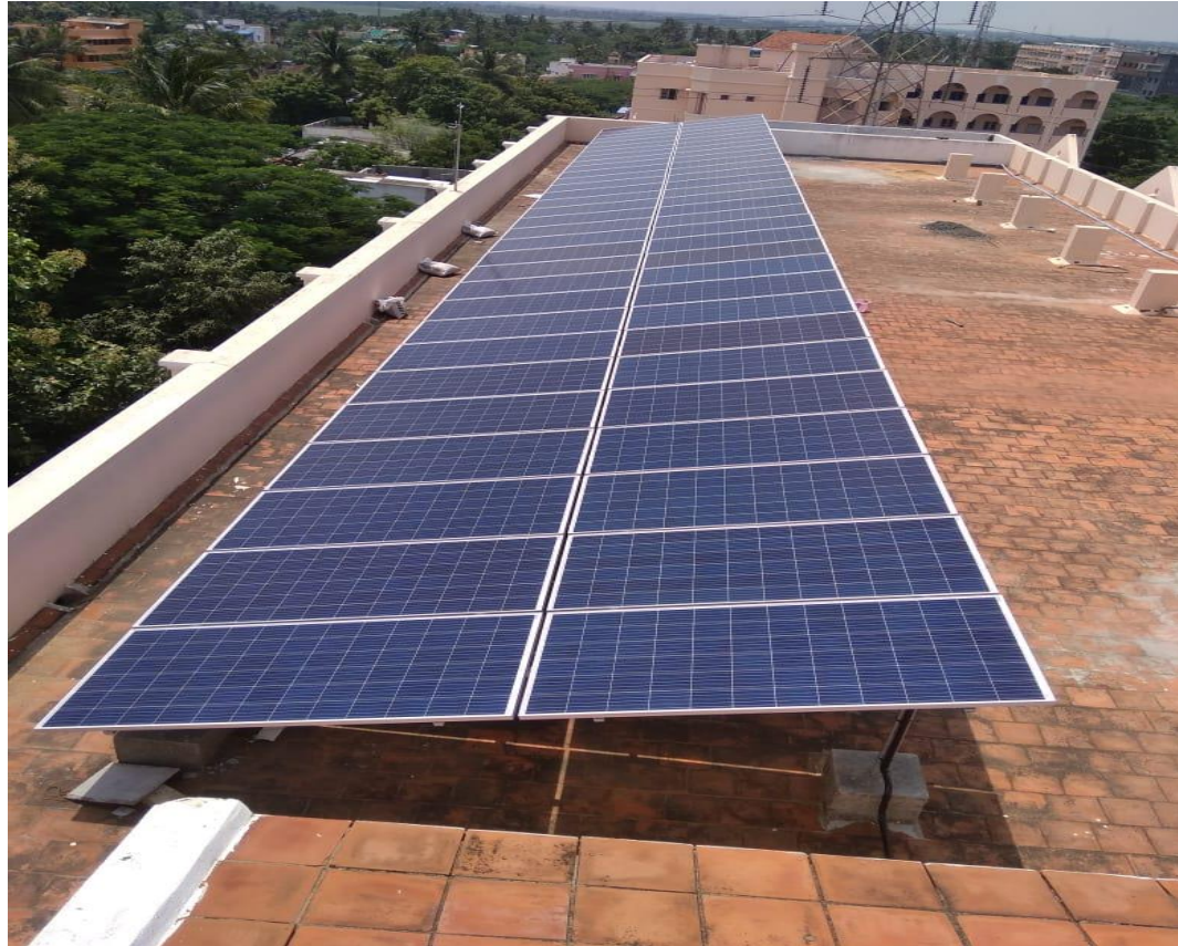
SOLAR POWER INVERTER
